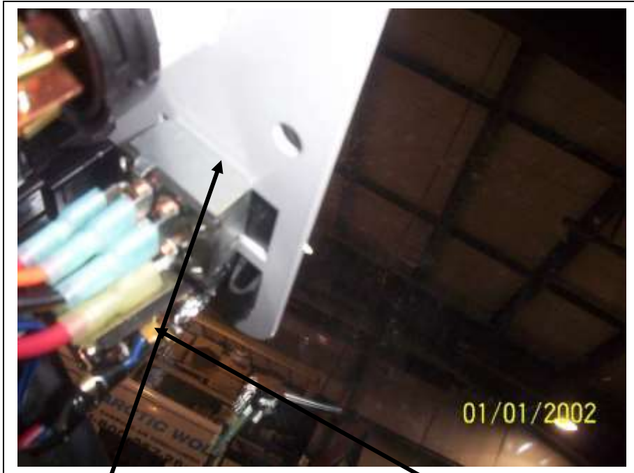
Blower switch mounted on console
