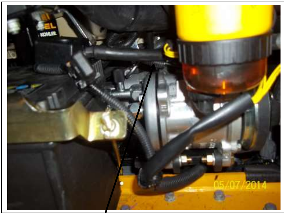
Electrical connections at compressor. Wire from binary on the drier to the compressor clutch.
