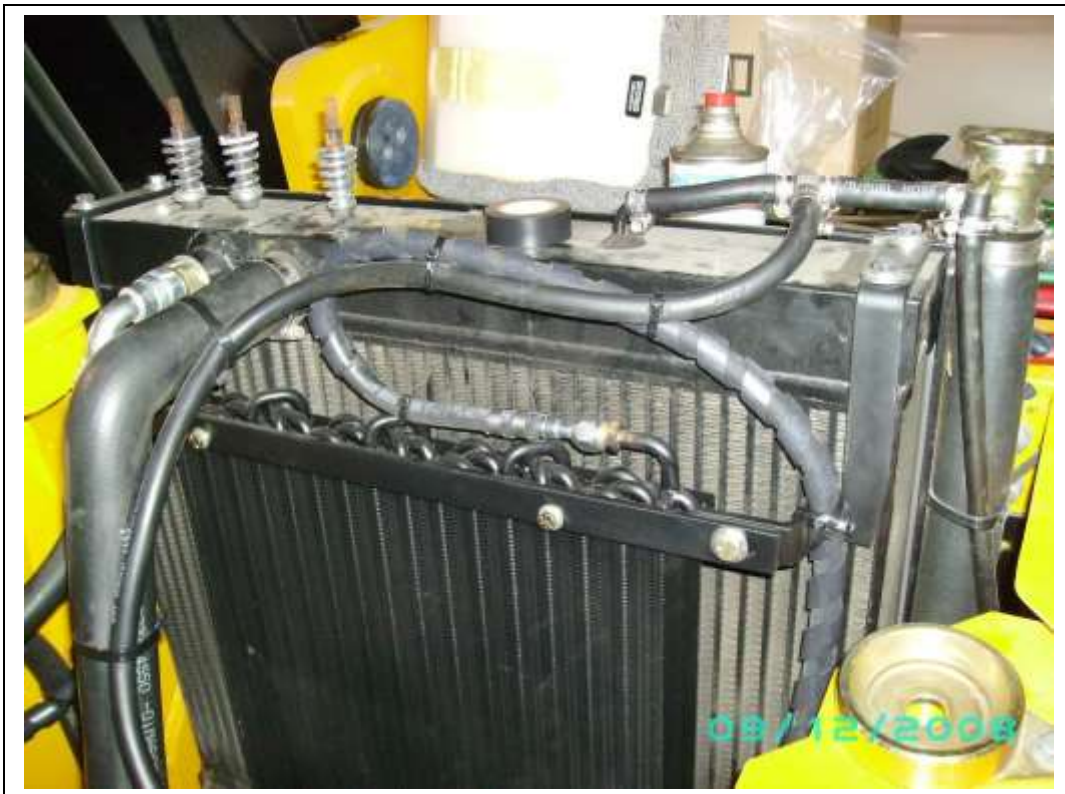
Hoses connected to the condenser. NOTE: Condenser is mounted differently.
